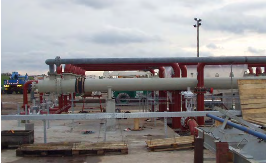
Figure 10 – Process fluid heat exchangers used in conjunction with cooling fans at Soultz, France.
