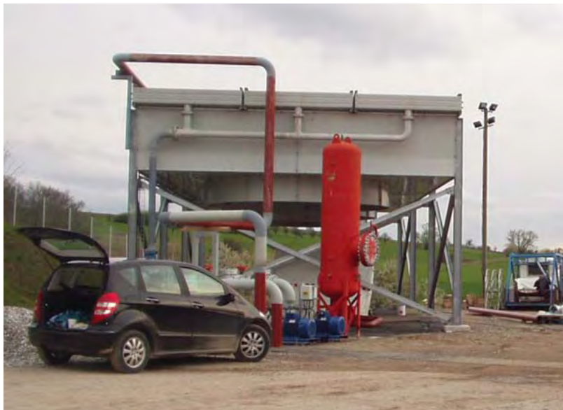
Figure 9 – Cooling fans used in EGS circulation testing at Soultz, France. Shown here prior to installation, these will be positioned over or adjacent to the heat exchangers for operation.
